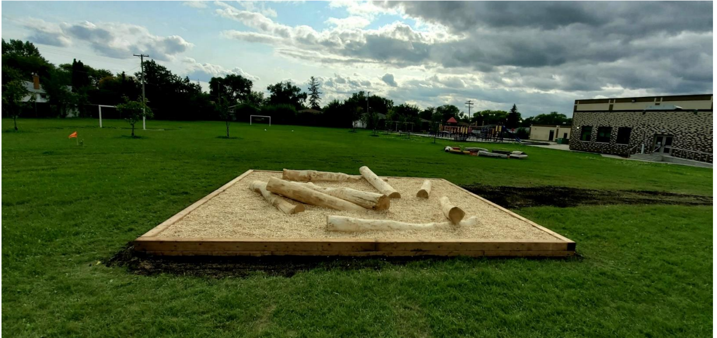
After 3 years of fundraising by our PAC, we are excited to announce the addition of this natural log play structure, located in the field behind our Circle Garden.
